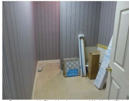
Rest room with Plumbing Issues and No Vanity/Sink
