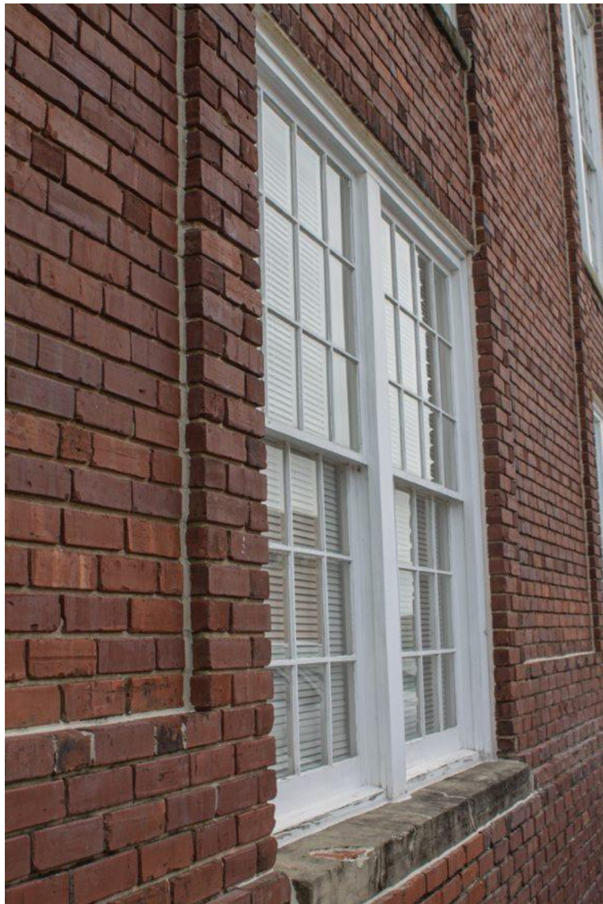
Photo 12 – North elevation detail. Note 1998-era windows, chipped, concrete-parged, masonry windowsill and caulking used in joint between wall face and in one-half-depth brick buttress/projection.
