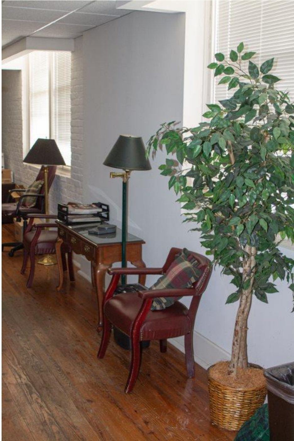
Photo 19 Northeast first-story office, looking north. Note exposed, painted masonry wall, and sheetrock wall section.
