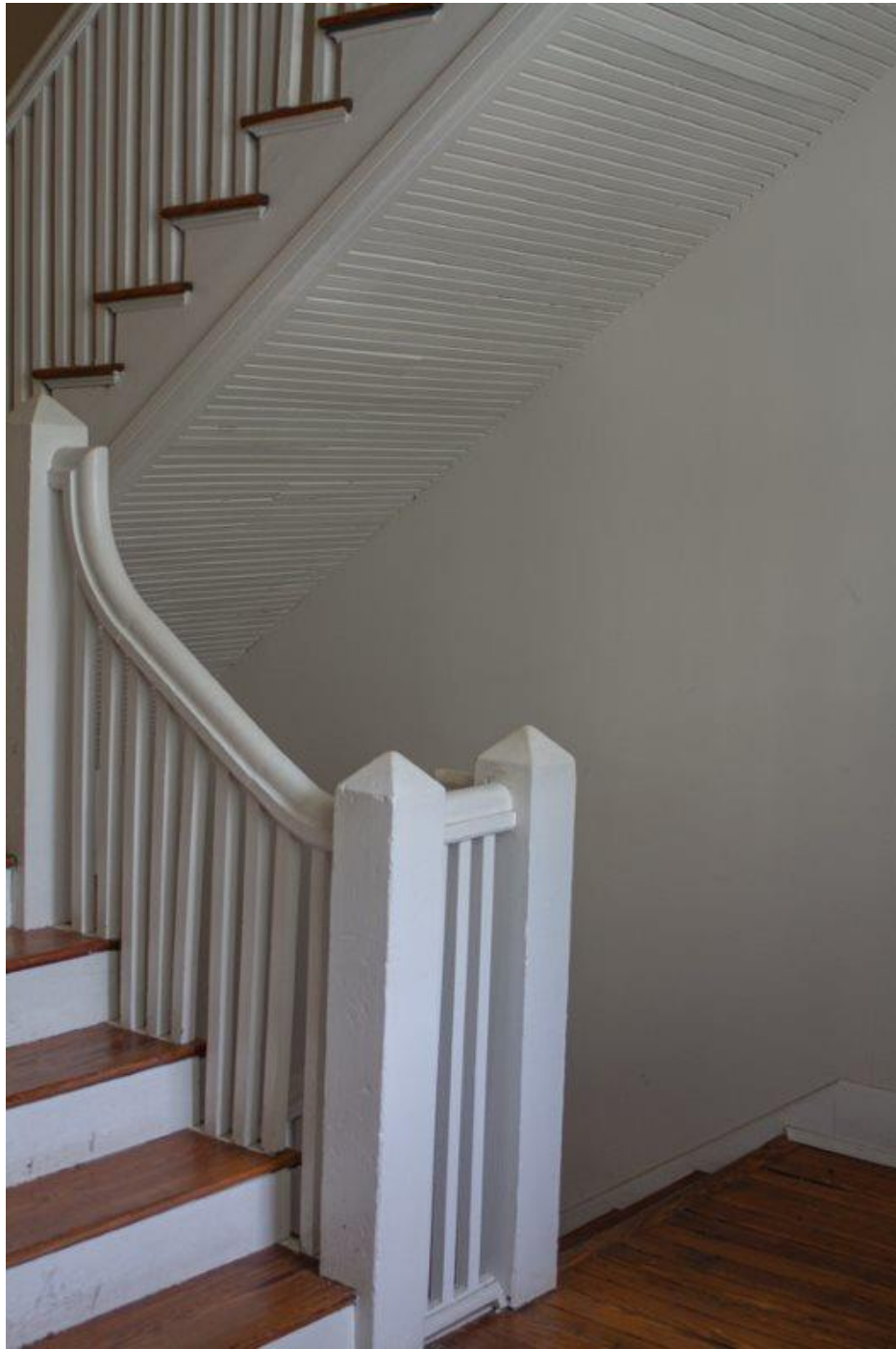
Photo 25 Second-story landing. Note original hardwood floors and staircase details including newel posts, balusters, and handrails.
