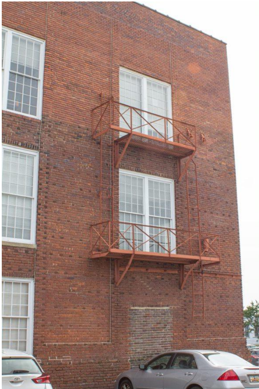
Photo 14 North elevation detail. Note ca.-1933 fire escape and visually contrasting, early masonry infill on first story and steel L-angle structural supplemental support.
