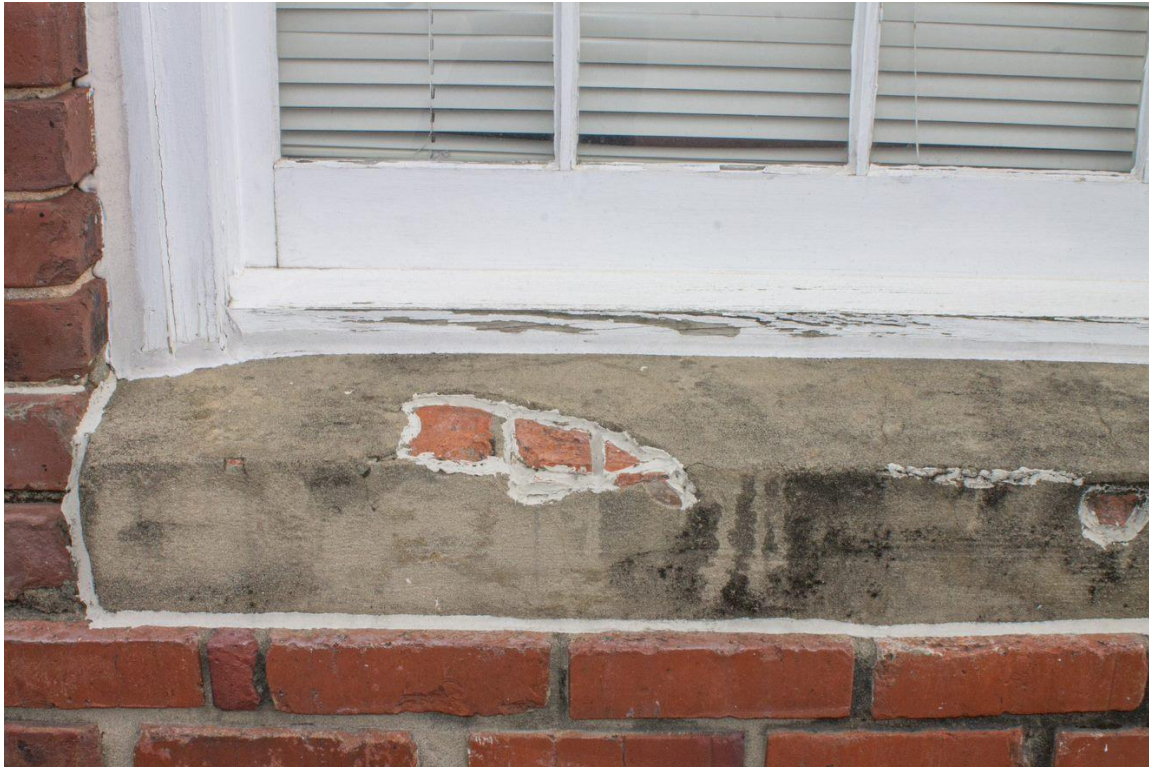
Photo 13 North elevation detail. Note 1998-era wood window and chipped, concrete-parged, masonry windowsill.
