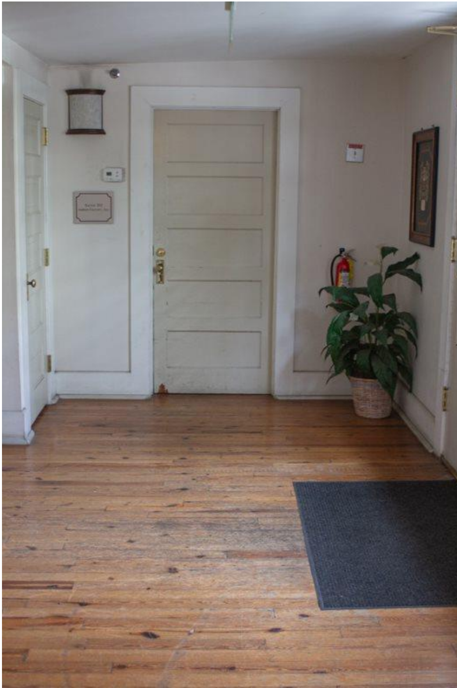
Photo 24 Northeast first-story office entry from front hallway, taken from the perspective of the southeast office entrance looking north. Note original hardwood floors and five-panel, 1930s-era door to storage closet under staircase.
