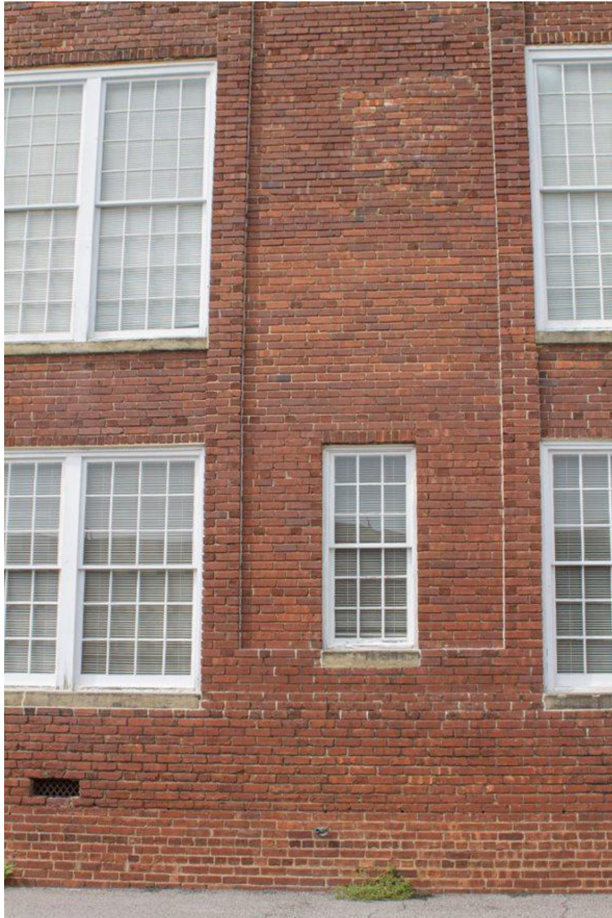
Photo 8 – South elevation illustrating general 1998-era window composition and appearance and singular exceptional window. Note 7/1 Flemish bond brick pattern with contrasting headers to stretchers and discoloration from earlier masonry patching between second-story windows.
