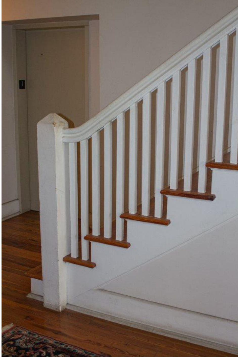
Photo 18 Front entrance detail, taken from the perspective of the southeast, looking north. Note original floorboards and historic staircase.
