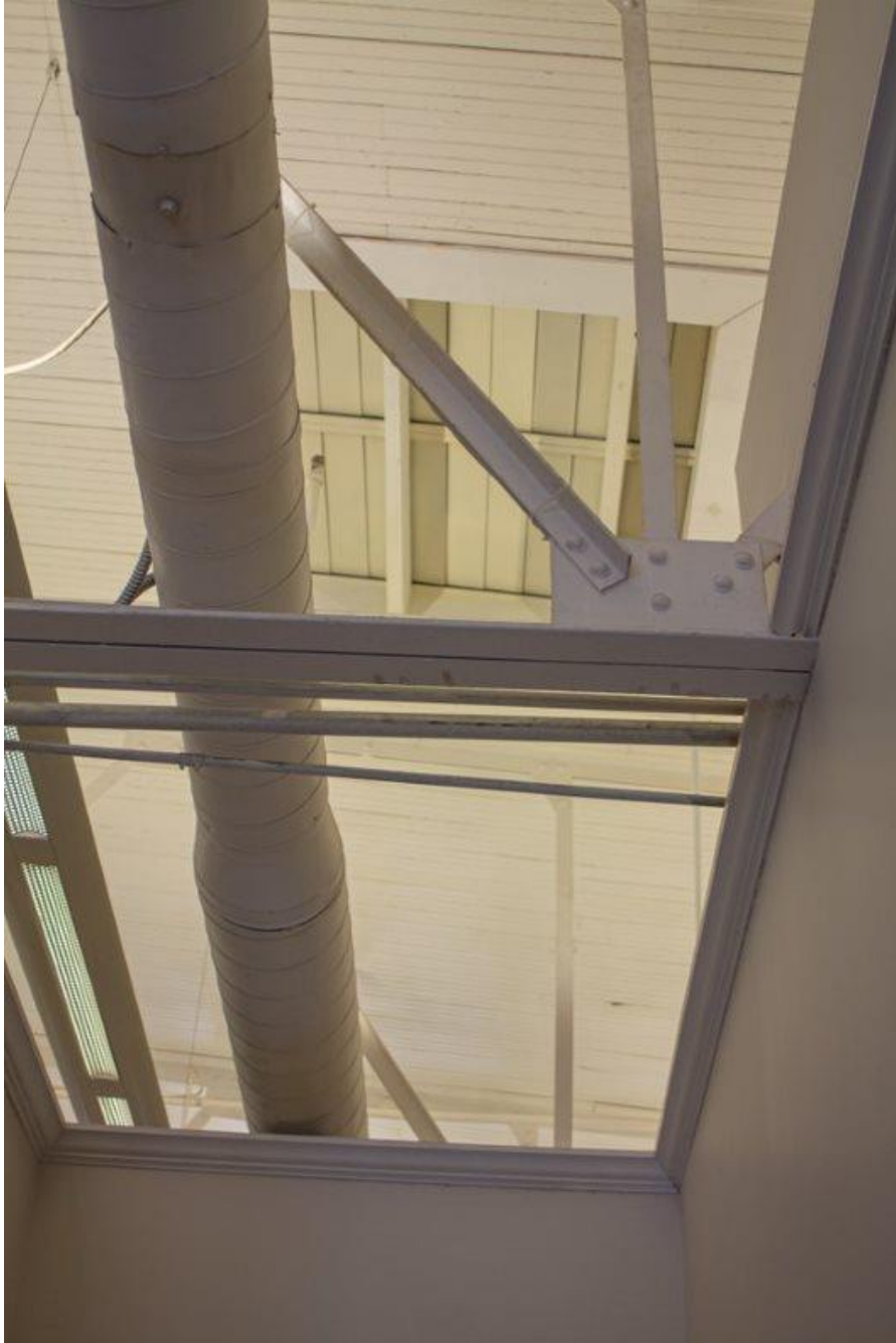
Photo 37 Third-story central office ceiling detail. Note steel bow truss configuration, exposed HVAC ductwork beadboard ceiling, roof scuttle, and ca.-1998 era sheetrock walls and trim.
