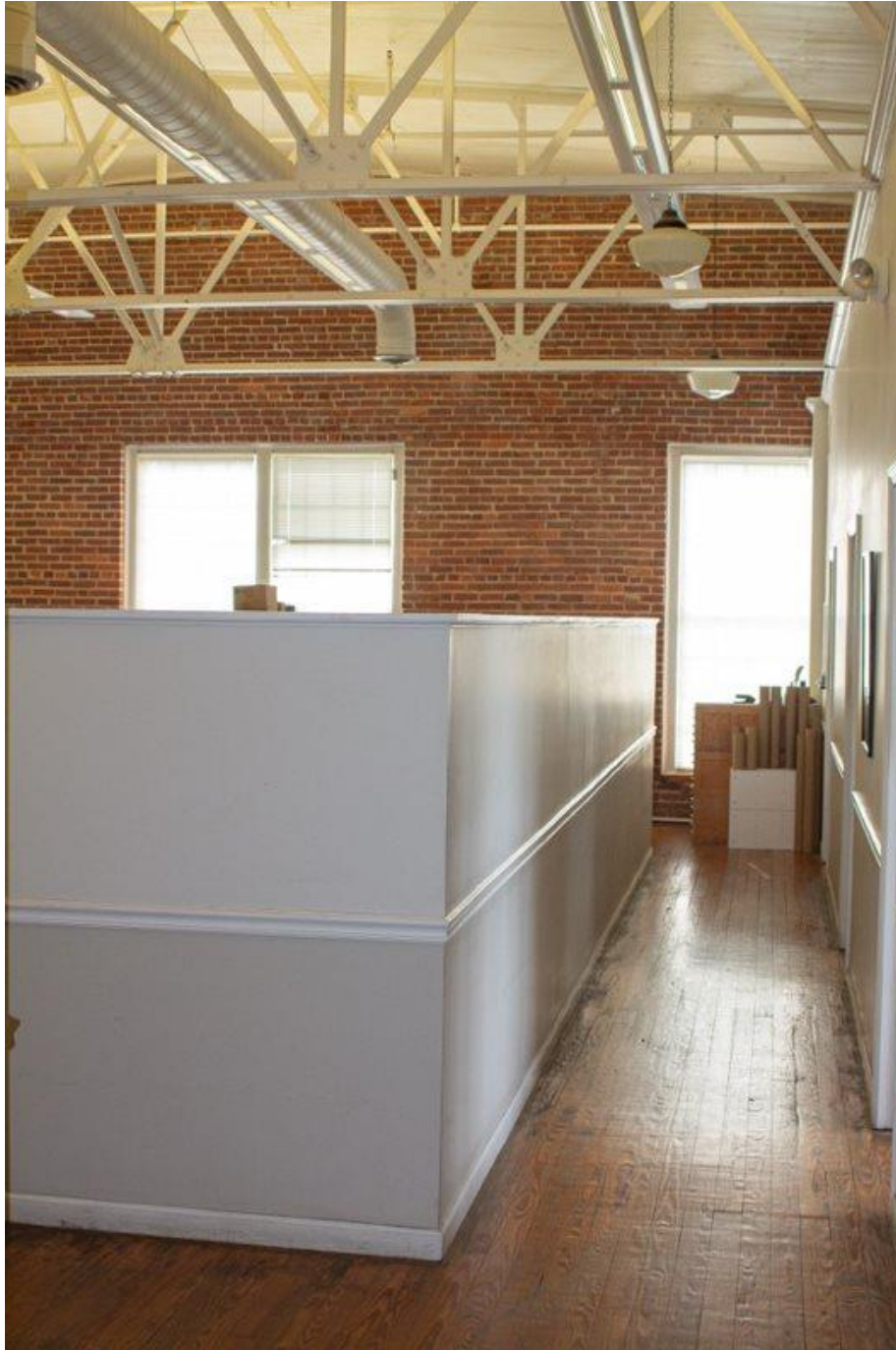
Photo 35 Third-story central office general conditions. Note steel bow-truss details, exposed masonry wall and original hardwood flooring.
