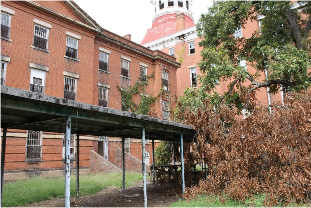
15. Rear of first southern north/south wing and center block, view to the northwest
