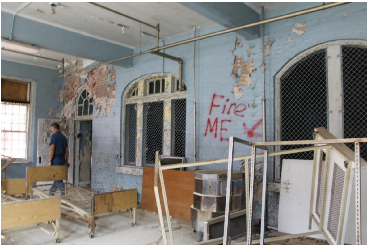
48. Northern section, east/west block, former exterior wall now in sunroom, view to the northwest
