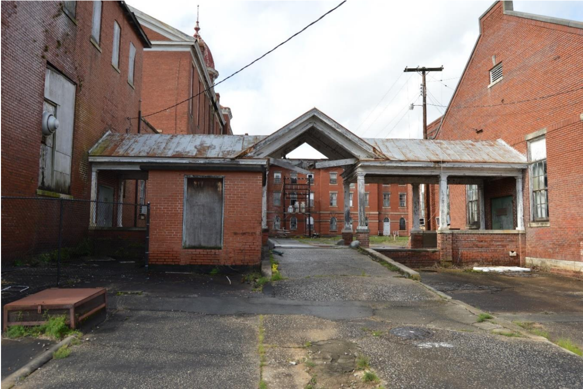
67. Rear view of hyphen between center kitchen wing and women's dining hall, view to the west
