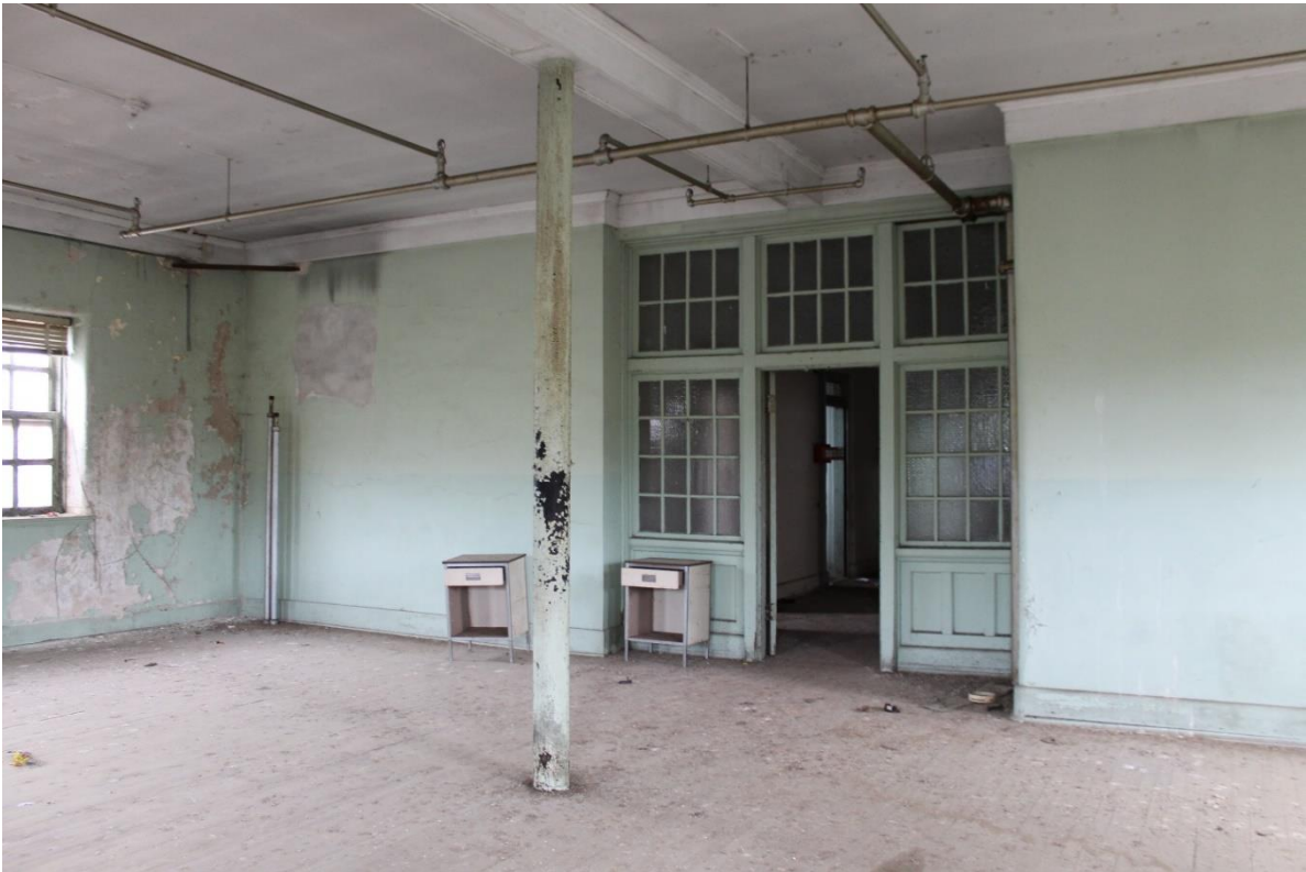
54. Southern east/west terminal block, upper level front room, view to the northeast
