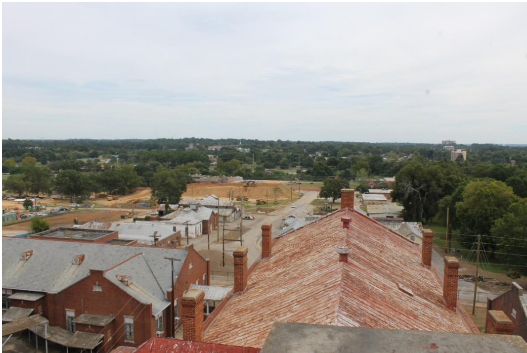
26. Center section roof with women's dining hall on left, view to the east
