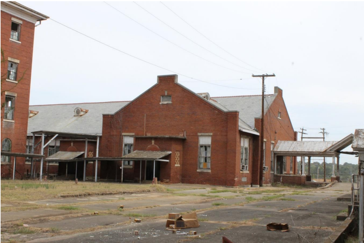
68. Women's dining hall, front (west side) and south end, view to the east
