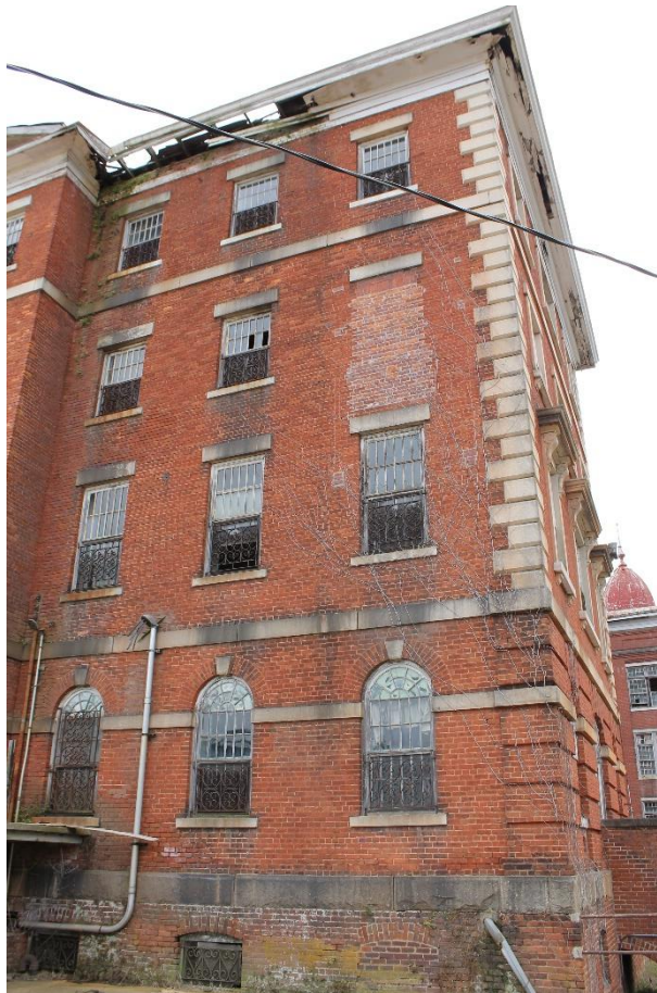
6. Northern terminal east/west block, north side and front, view to the south
