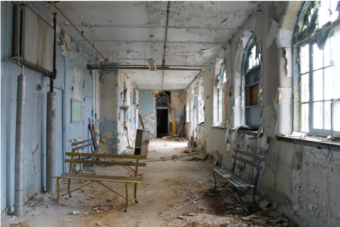
50. Northern section, sunporch added across rear of north/south wing, view to the north
