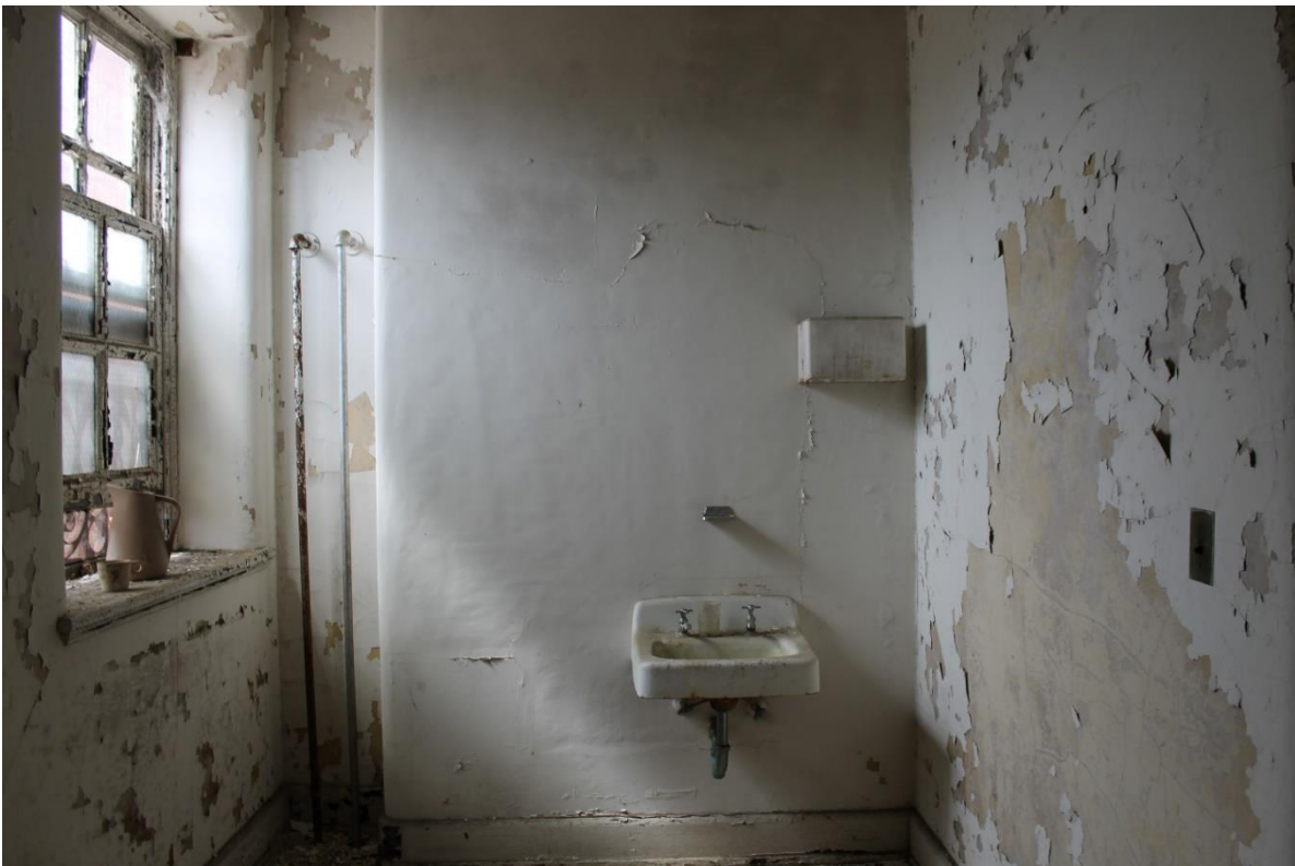
56. Southern east/west terminal block, upper level, typical individual room, view to the east
