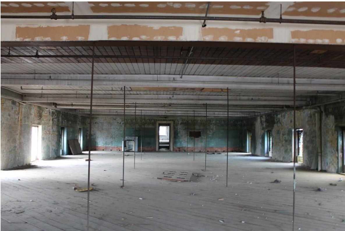
40. Center block, 4 th floor looking to the rear, view to the east
