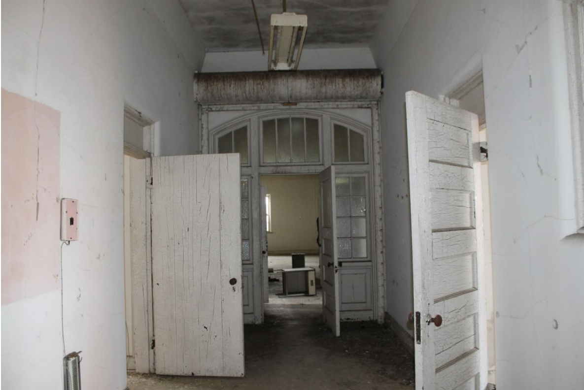
55. Southern east/west terminal block, upper level middle section looking to the rear, view to the east
