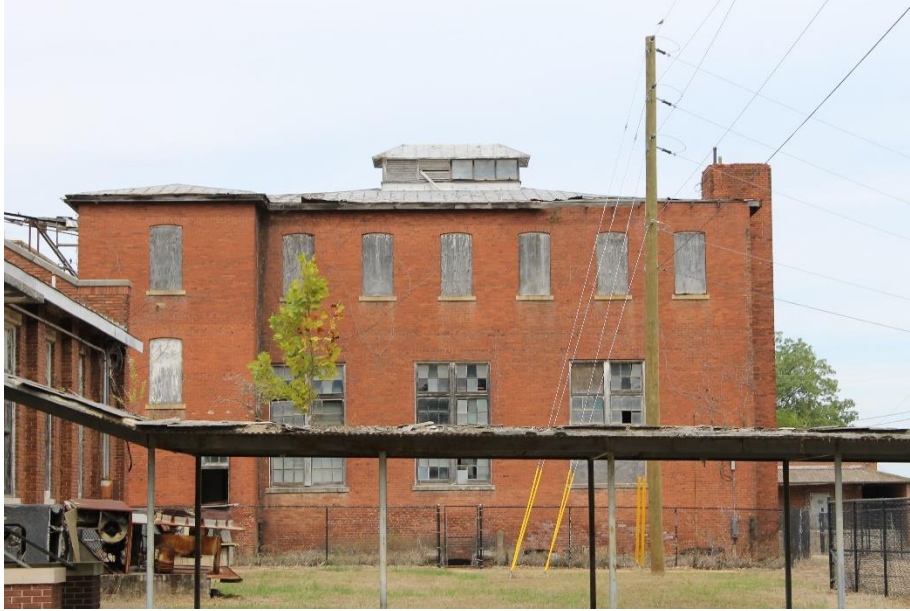
17. Southern side of center block – rear kitchen/laundry wing, view to the north
