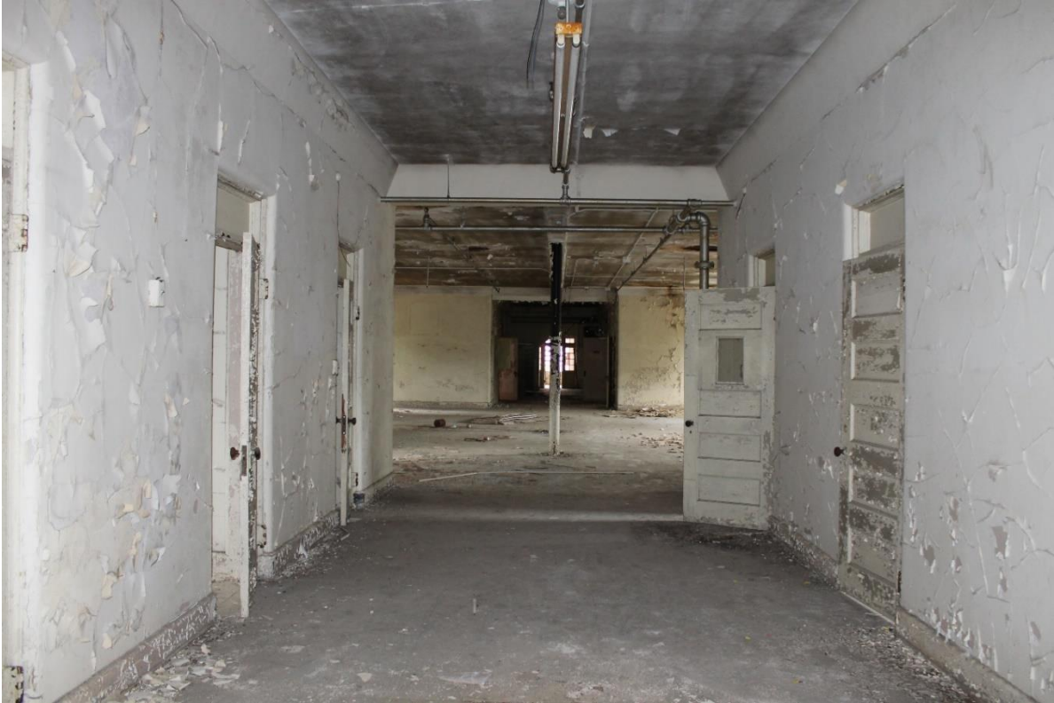
59. Southern north/south wing, upper level, looking towards 1915 ward, view to the north
