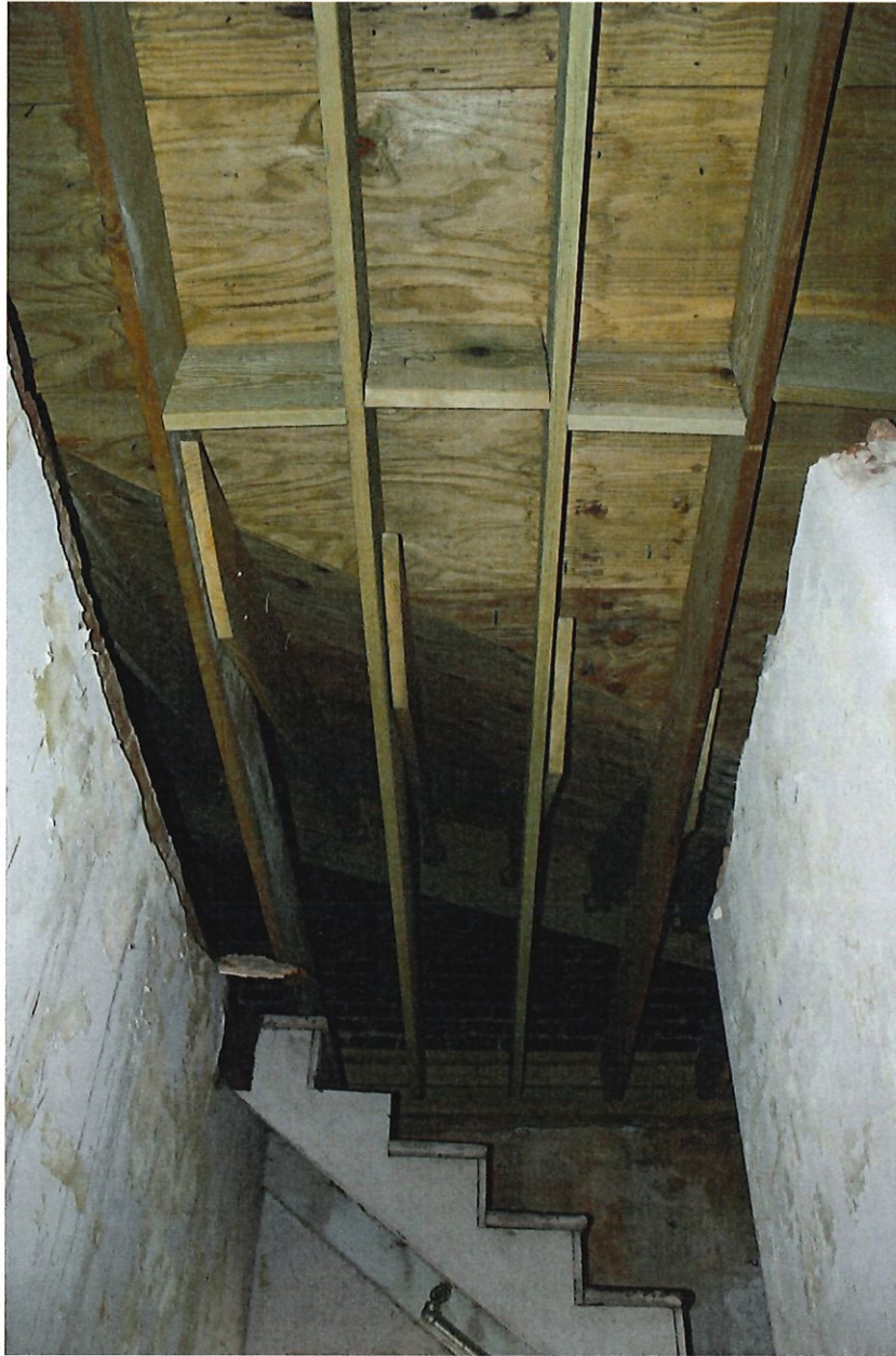
Photo 4 – Babcock Building 2150 Bull St. Columbia, SC New joists and ceiling system in stairwell 8/15/2019
