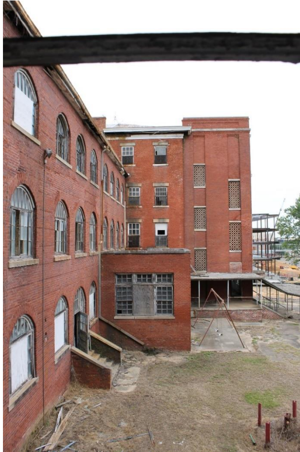
25. Rear (east side) of second (northernmost) east/west wing, view to the north
