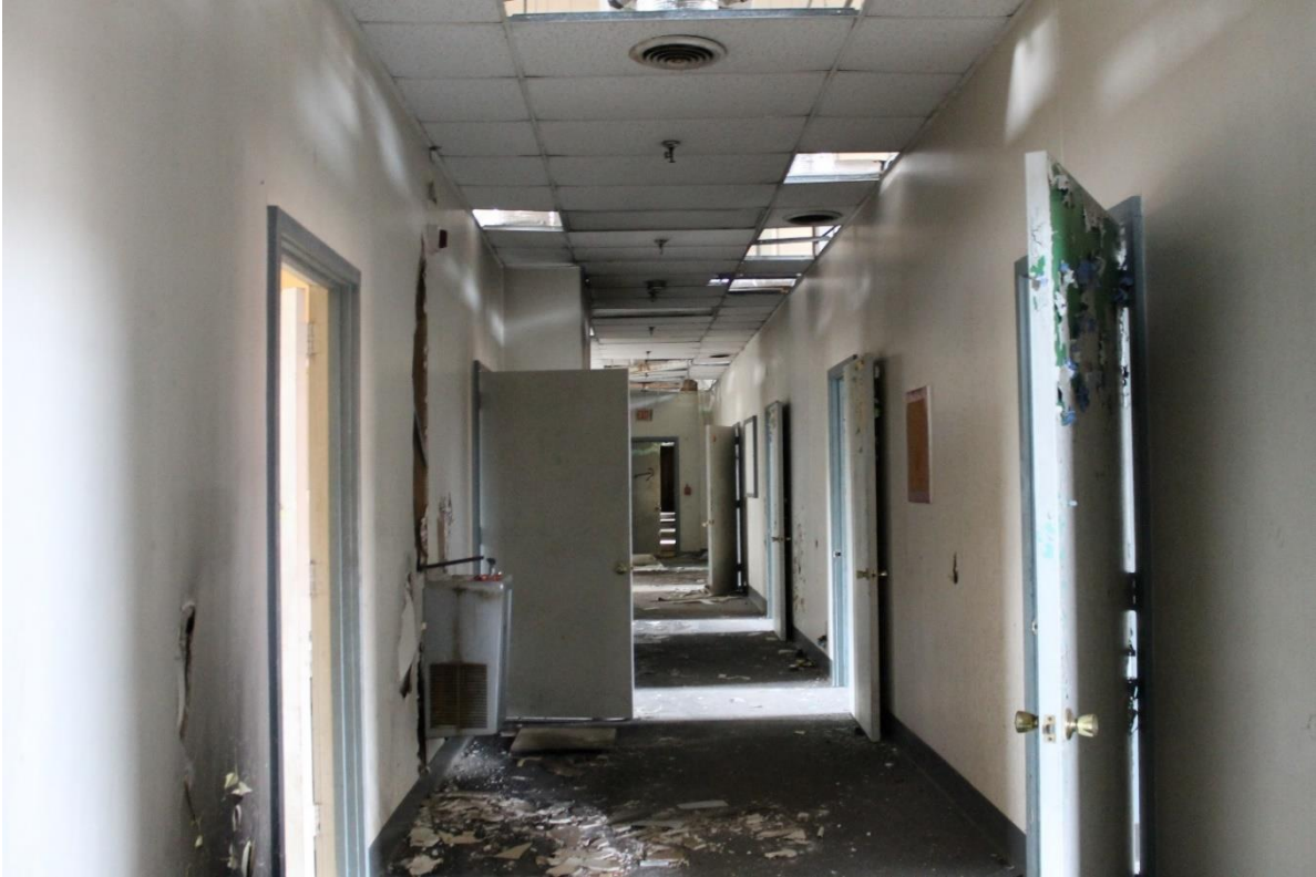
37. Center block, 3 rd floor looking to the rear, view to the east
