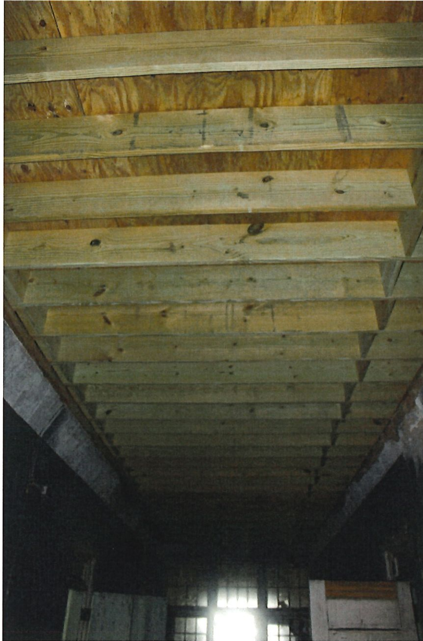
Photo 2 – Babcock Building 2150 Bull St. Columbia, SC New ceiling joists where originals burned, third floor ceiling, southeast section of building 8/15/2019
