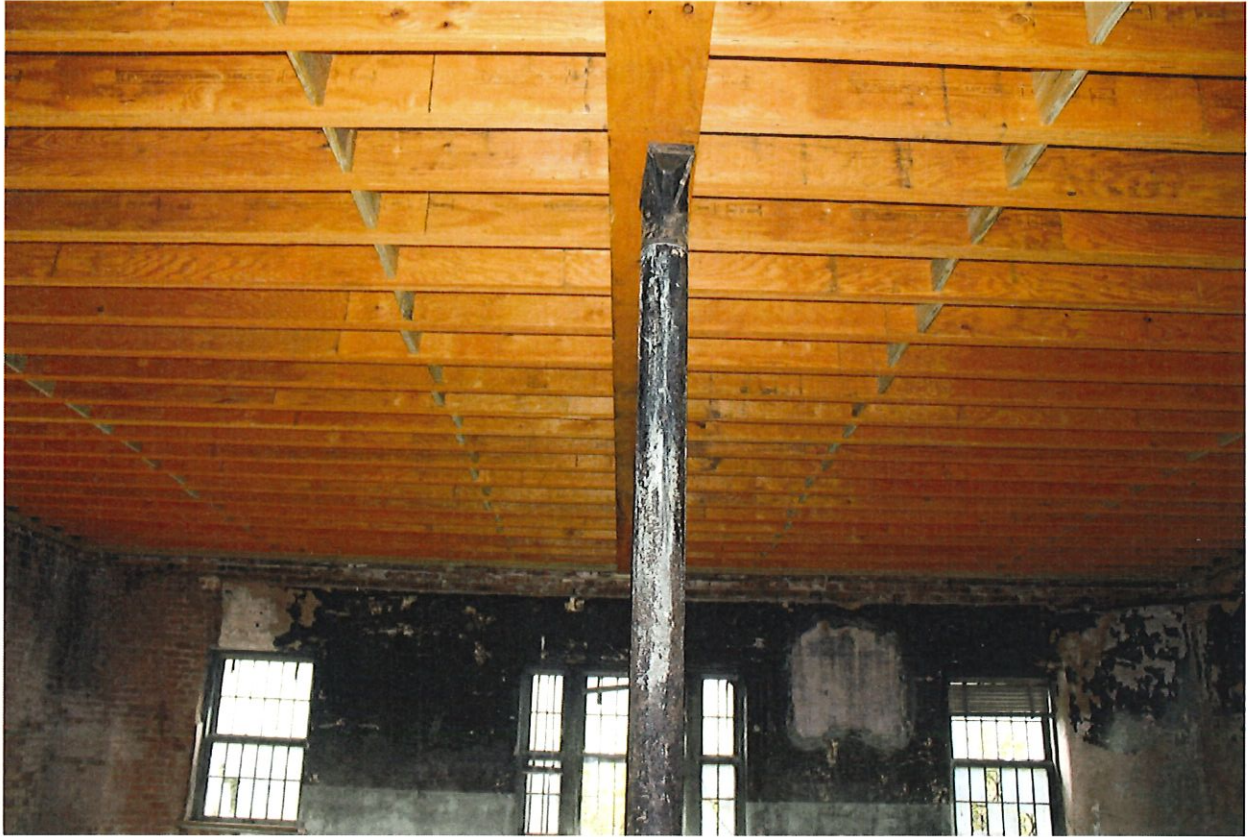
Photo 3 – Babcock Building 2150 Bull St. Columbia, SC New third floor ceiling joists replacing burned joists 8/15/2019
