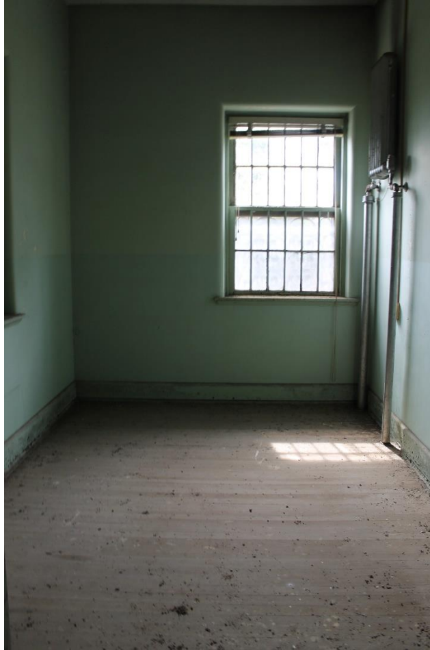
57. Southern east/west terminal block, upper level, typical individual room, view to the north
