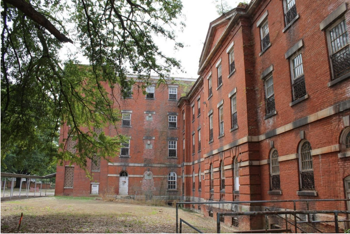
13. Northern side of southern terminal east/west block and rear (east side) of north/south wing, view to the southwest
