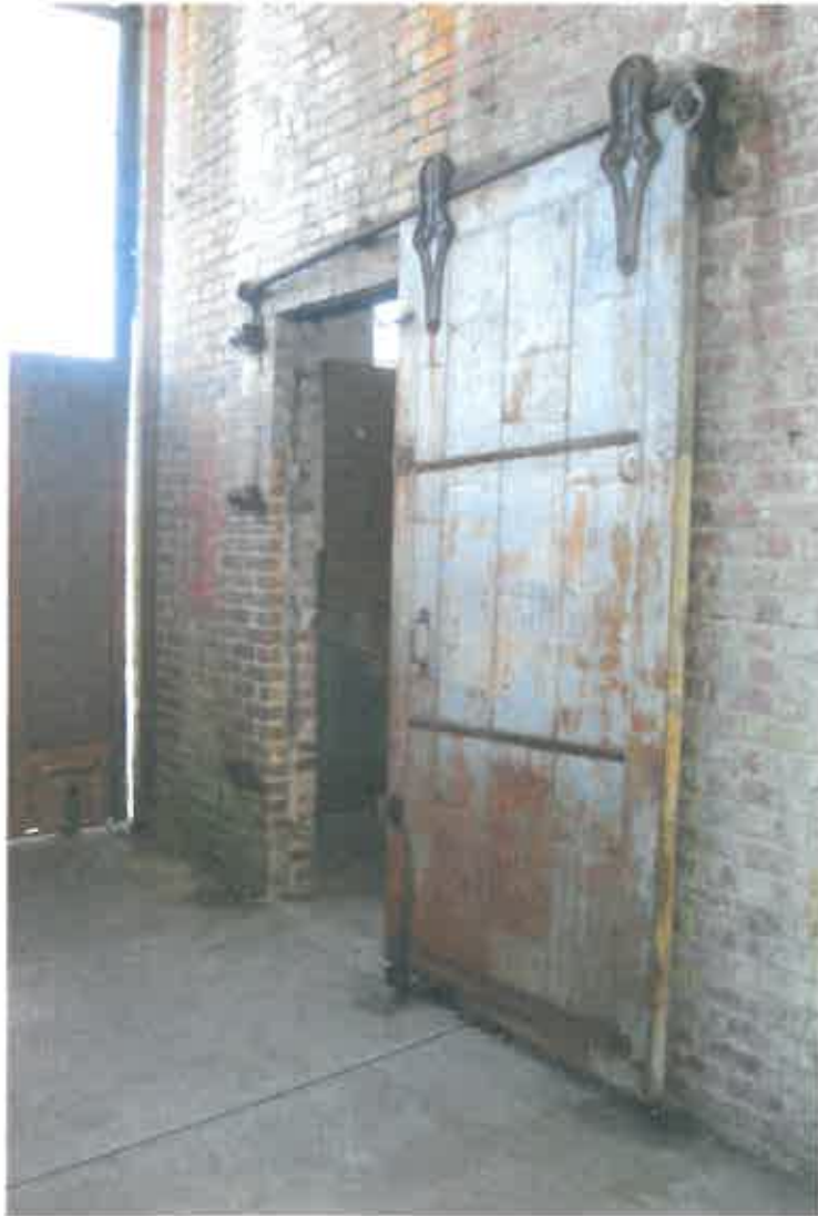
Photo 15 – Interior fireproof door
