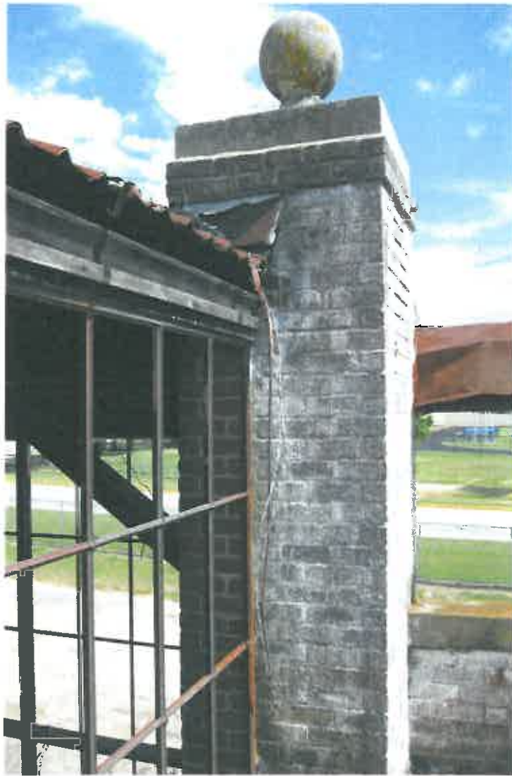
Photo 23 – Concrete finial, southwest corner
