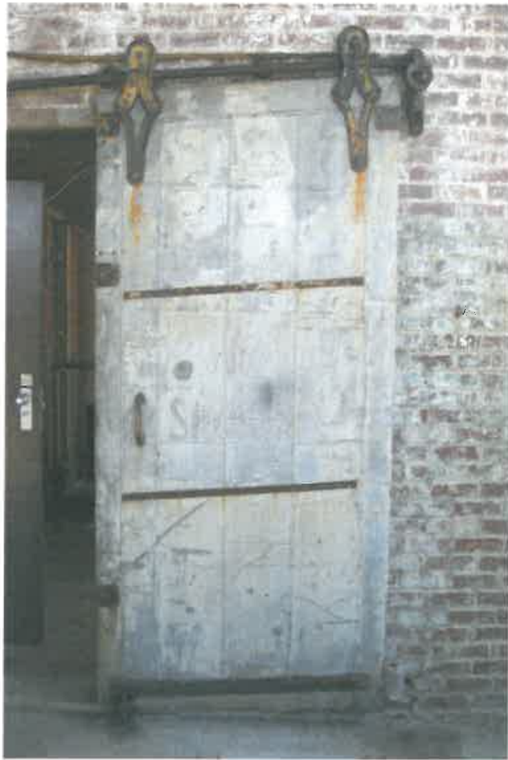
Photo 14 – Interior fireproof door
