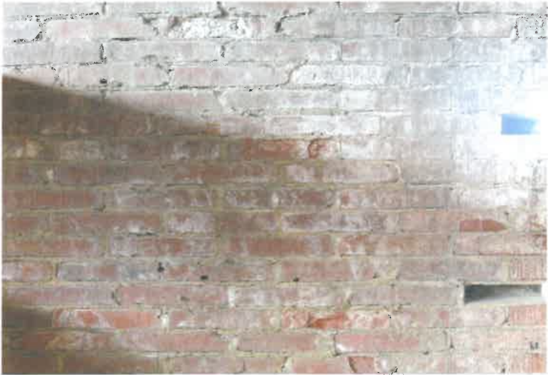
Photo 13 – Interior brick detail, repointing needed
