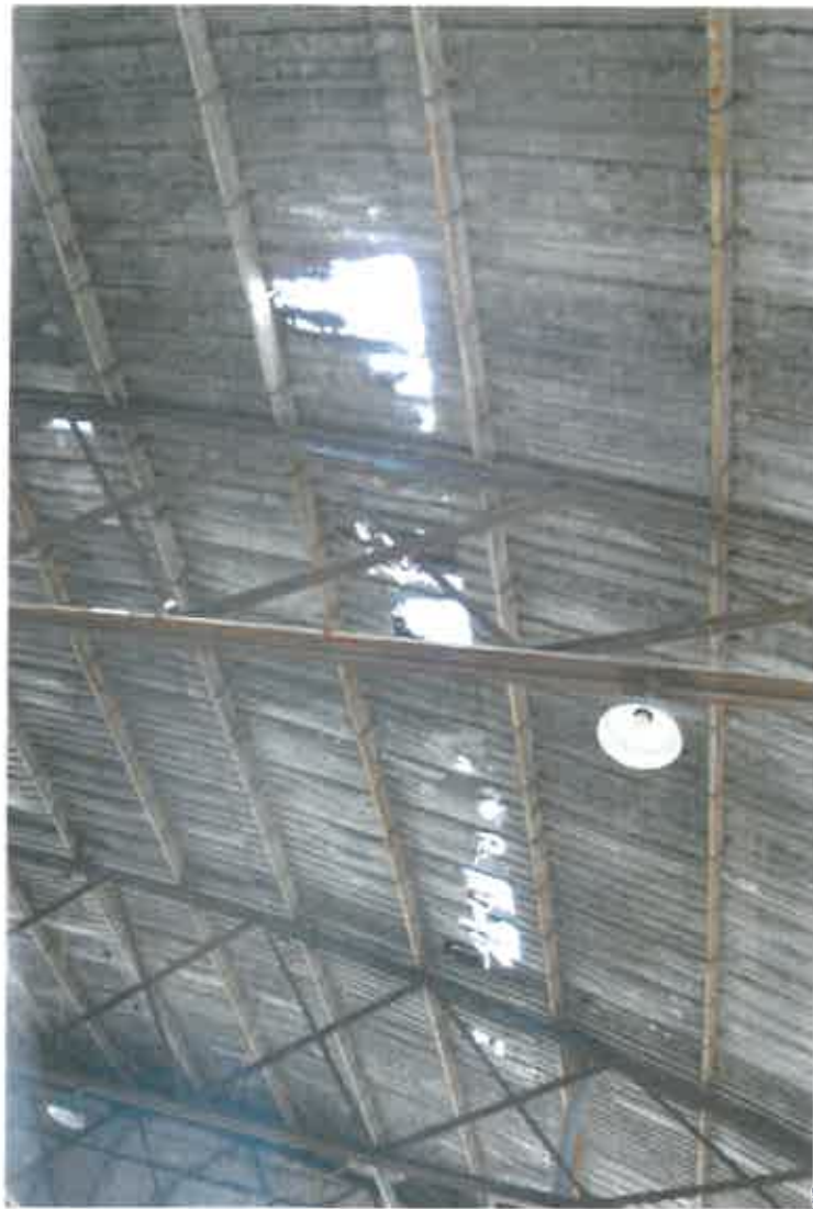
Photo 31 – Roof deterioration and exposed trusses
