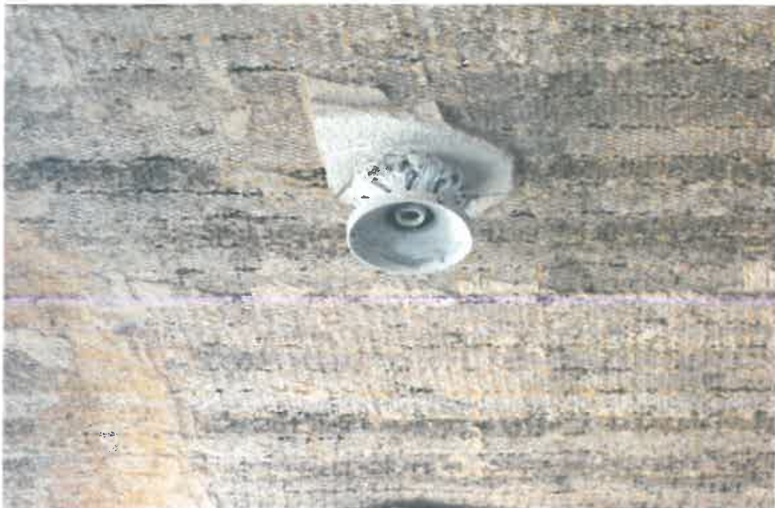
Photo 36 – Bathroom light fixtures
