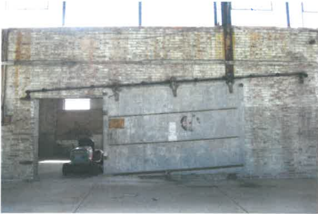
Photo 16 – Interior fireproof door
