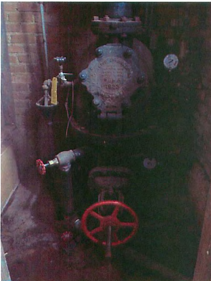
Photo 12: Existing fire protection riser.
