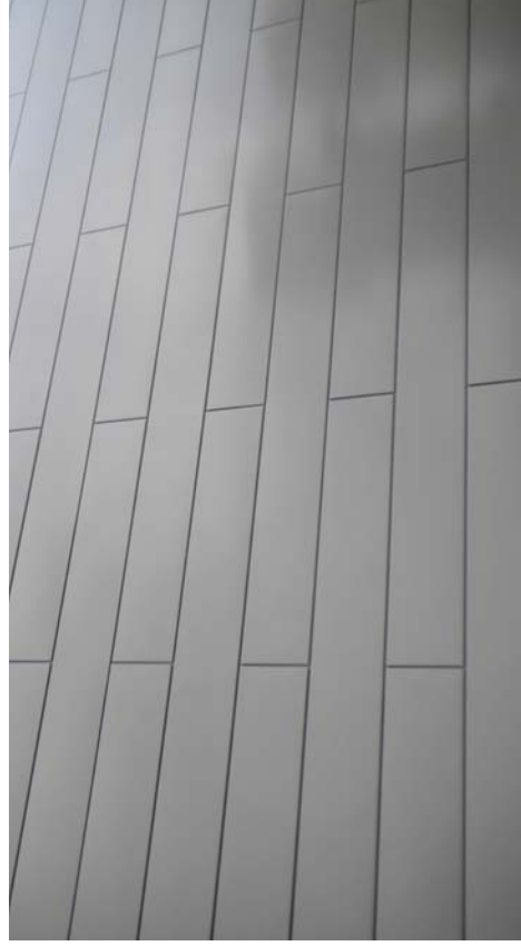
MTL-1 GARLAND ELEMENT MATERIAL HORIZ ARCH WALL PANEL SYSTEM W/ CONCEALED FASTENERS COLOR: PEWTER STAGGERED JOINTS
